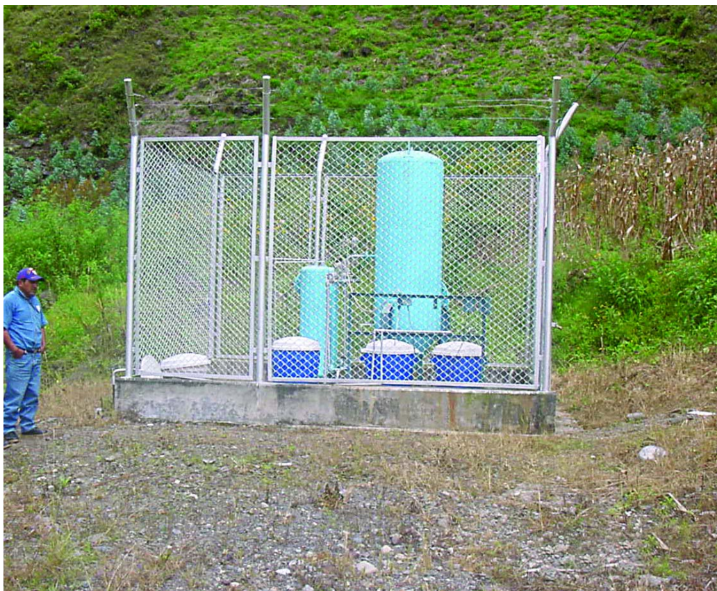
Monitoreo de Calidad de Agua Potable Drink Water quality monitoring
