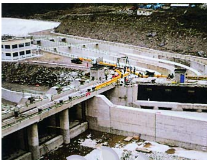
Lote 1: Obras concluidas de cabecera de la C.H. San Gabán II. Lot 1: Concluded head works of the San Gabán II Hydroelectric Power Plant.
