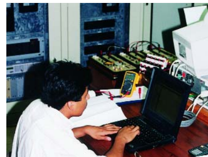
Centro de control San Gabán II. Control centre San Gabán II.
