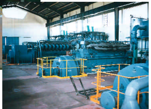
Sala de Máquinas, Taparachi Power House, Taparachi
